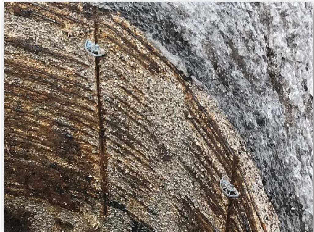
Armatures visibles, corrosion > 5 cm
